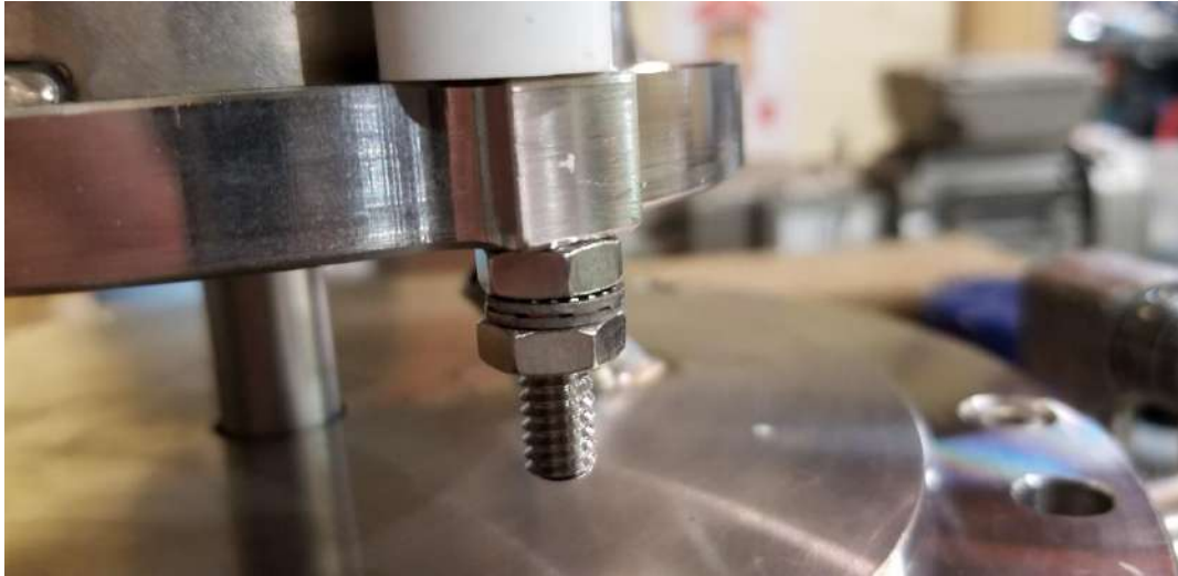
Fig 12. The proper hardware assembly to re-install the roller rods as shown. Jam nut – Wedge “nord” lock washer – jam nut.
